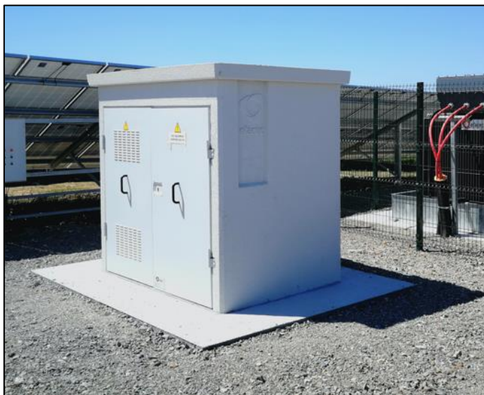
Plate 4-7. Outdoor cabin switchgear
