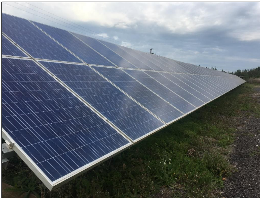
Plate 4-3. Solar panels with south facing configuration
