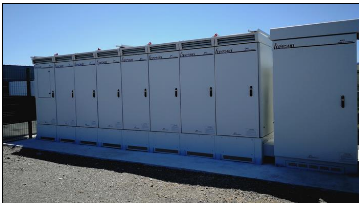
Plate 4-4. Typical outdoor centralised inverter
