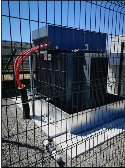
Plate 4-6. Typical outdoor transformer
