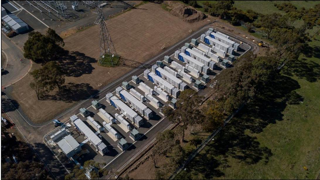
Plate 4-8. Typical battery storage compound configuration ( image reproduced courtesy of Fluence Energy ).
